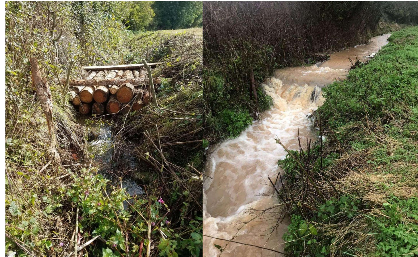
An example of a longitudinal leaky dam in the watercourse. Dam designed to retain water in channel. LEFT: on completion (Oct 19) RIGHT: during Storm Dennis (Feb 20)
