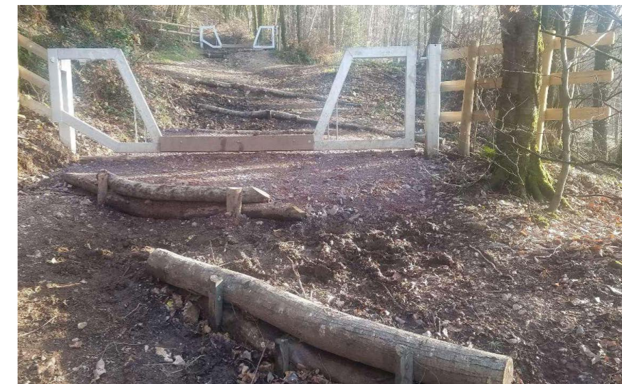
Example of the woodland tracks where heavy erosion and 4x4 use was contributing to sediment run off and overland flow. Closure of path to vehicles under a DCC issued Flood Prevention Order and installation of horse-friendly barriers & natural 'grips' to send water into the woodland floor.
